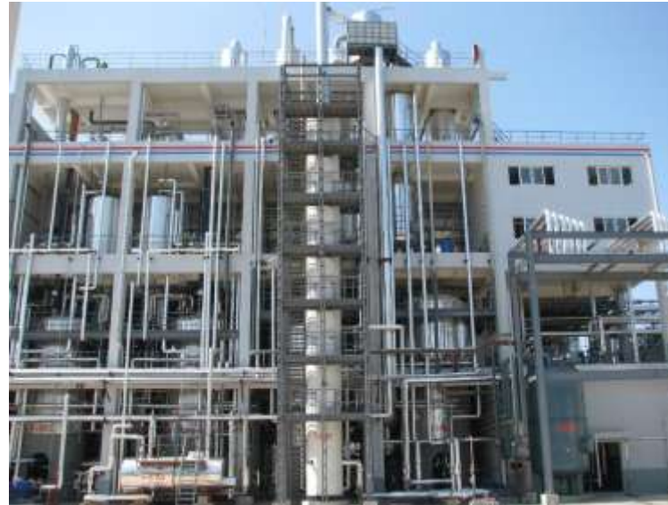
The main process reactor
