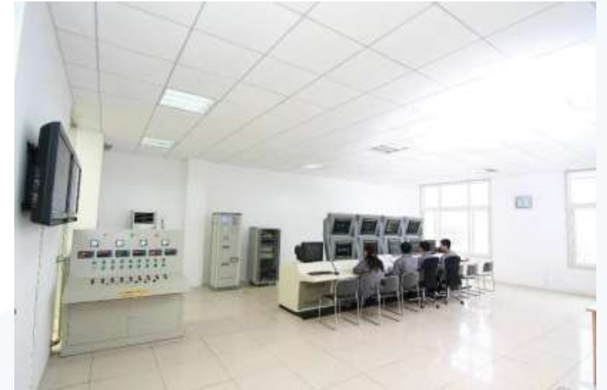
Main control room
